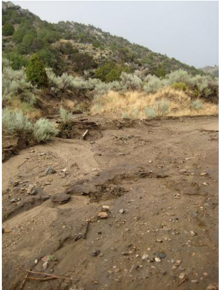
Figure 7: Erosion point feature on the Ramshorn Cr. Road created by high flow event. Image source: Breanne Bornemann.
