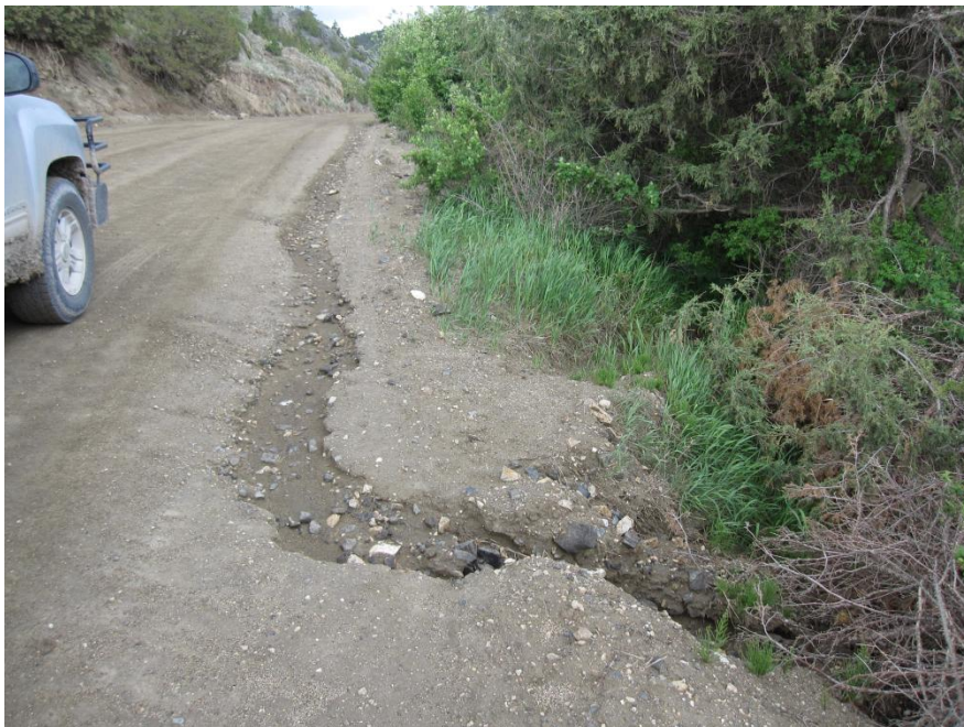
Figure 8. Upper Stone Creek. A storm event erodes the roadway into Stone Creek. (Photo, June 2013)
