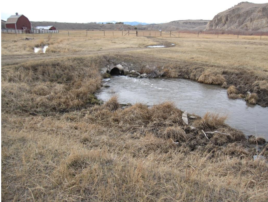
Figure 7. Lower Spring Creek. A new bridge is needed to replace the perched culvert to reduce sediment delivery and allow better fish passage. (Photo, November 2012)
